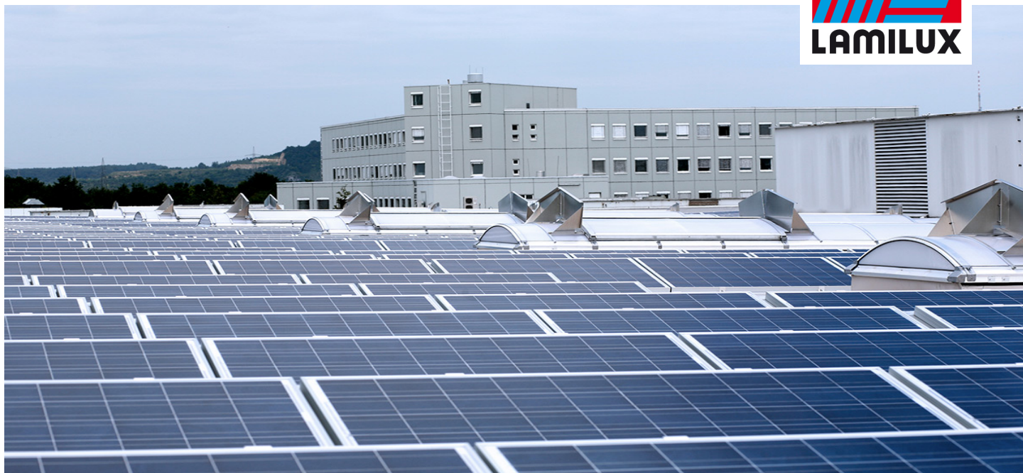
Schneider Electric, Regensburg, Germany
